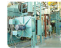
Figure 1. Two D-type 40,000 lb/hr watertube boilers equipped with economizers and a single 40,000 lb/hr, 12 MW electrode boiler were utilized to provide steam and high temperature hot water load at the John B. Shepherd Central Utility Plant.
